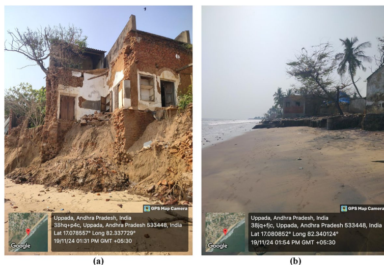
Fig. 21 Significantly eroded locations captured during field visits in location A (a) and location D (b) of Uppada Village. Source: Photographs were taken by the fifth author in Nov 2024 during the data collection
