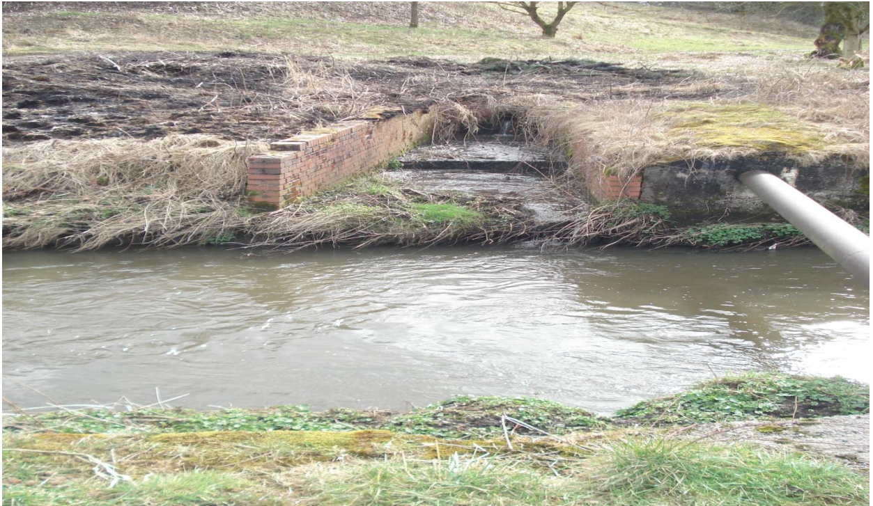
Fig. (8): Surface water discharge between locations 2 & 3, presumably from the housing development, south of the Golf course.
