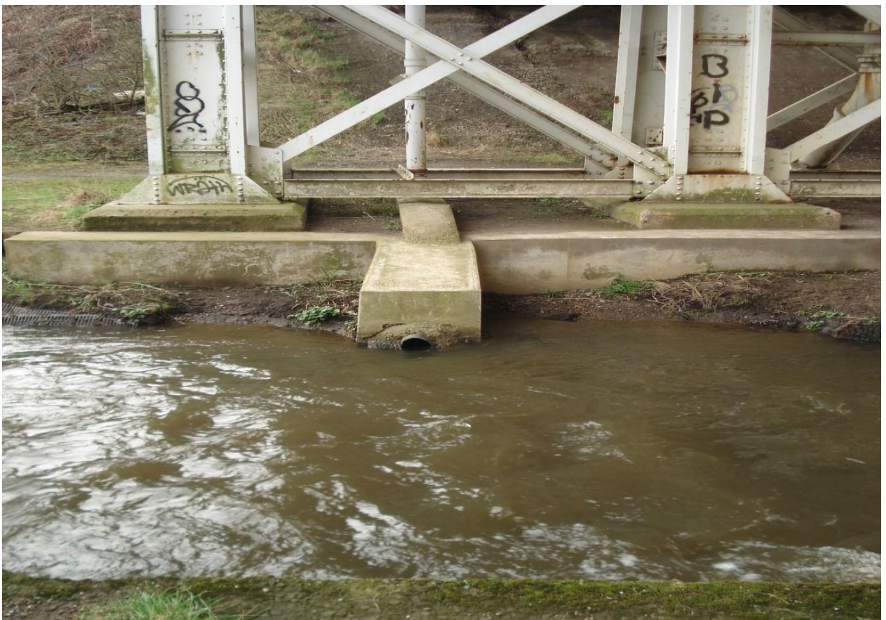
Fig. (5): Surface water discharge from Beaumont Road Bridge, approximately 25 yards east of Location 1.
